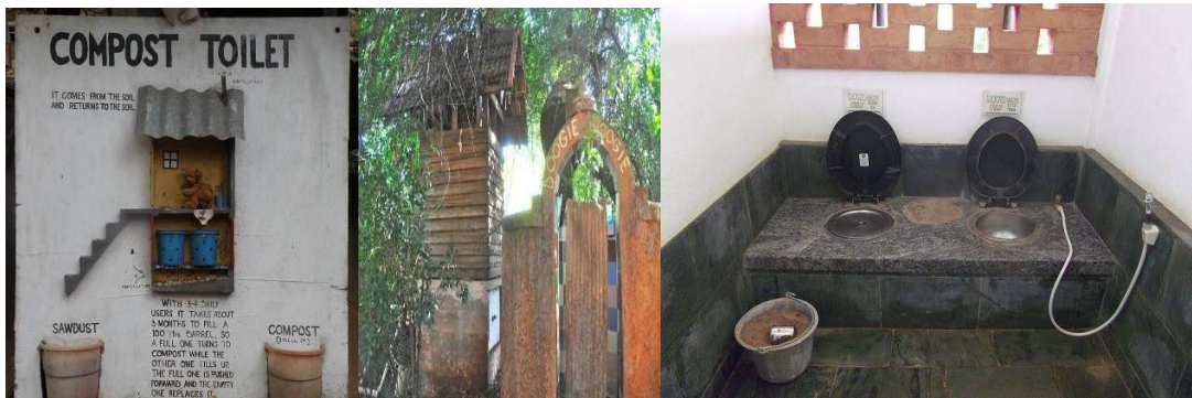
Figure 24. Compost Toilets in Fertile Forest and International House, Source: Personal and International House (International House 2011)
