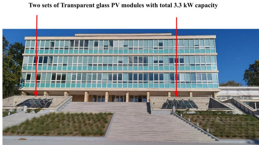
Fig. 3.4. A 3.3 kW transparent glass PV module at the entrance of the Aula building
